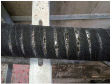
图1 电缆金属护套与绝缘外屏蔽层缺陷 Fig.1 Defect of metal sheath and insulation outer shielding layer of cable
