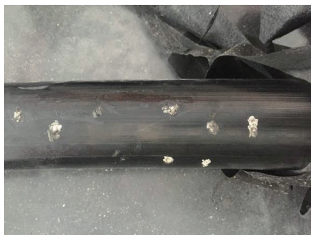
图 1 故障电缆外半导电层放电痕迹 Fig.1 Discharge traces of fault cable outside semiconducting layer
